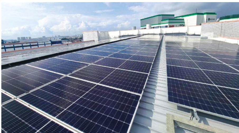
Installation of solar panels was completed at 10 property clusters, with a total generating capacity of 3,492 kilowatt peak.
