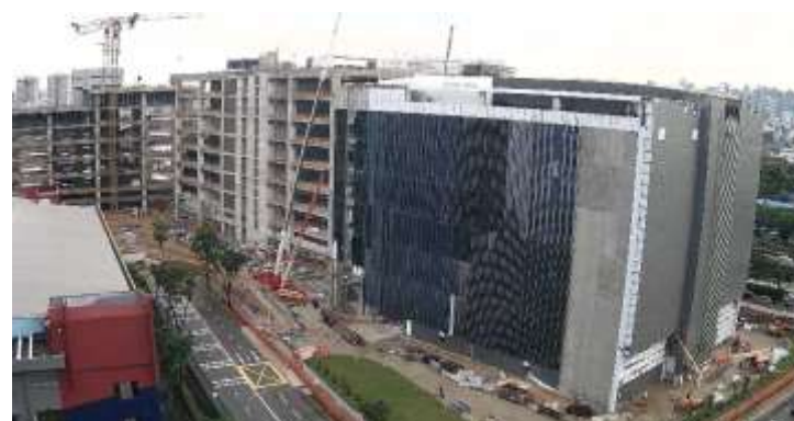
Block 165: Façade installation in progress; Block 163 and Block 161: Structural works in progress
