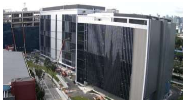
Completed structural works for all three blocks. Block 163 and Block 161: Façade installation in progress
